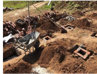
Brick column - no rebar
