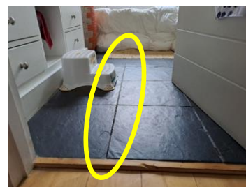
Cracked tiles in bathroom – on screed
