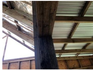
Affected timber door frame
