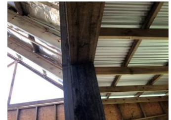
Affected timber section
