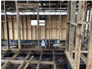
Damaged interior elements
