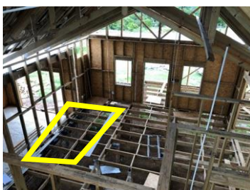
No concrete floor in kitchen
