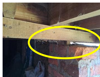
Timber deck not supported
