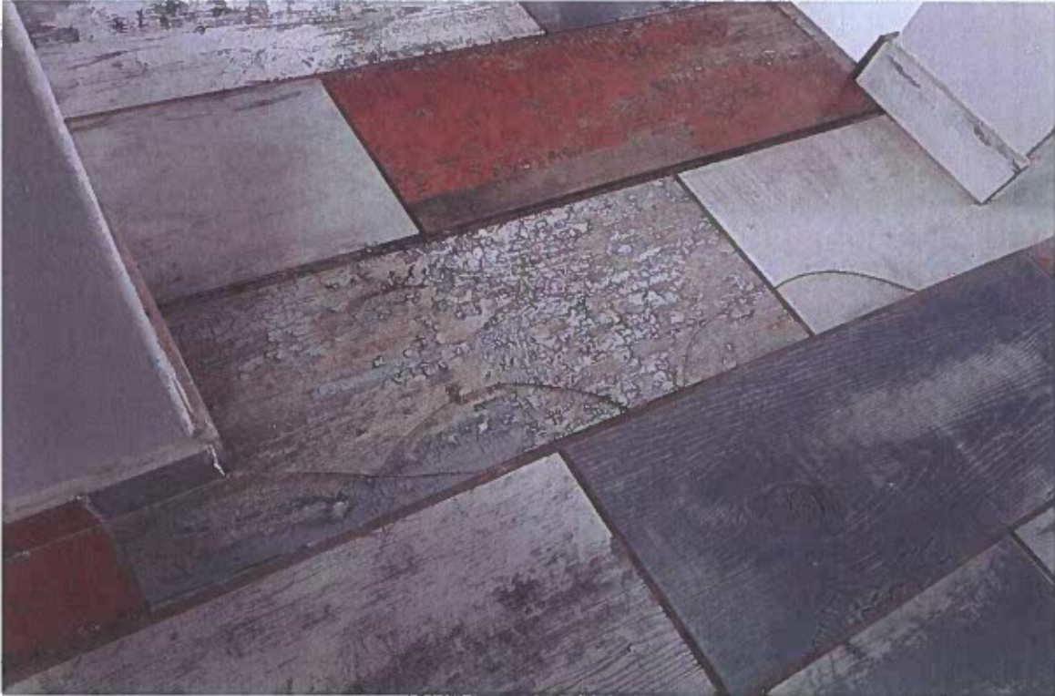
Plate 3 shows cracks on floor finish in the corrido..
