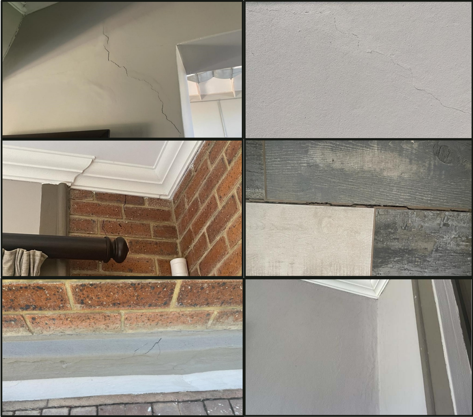
Figure 6: Showing structural cracks on the investigated house.
