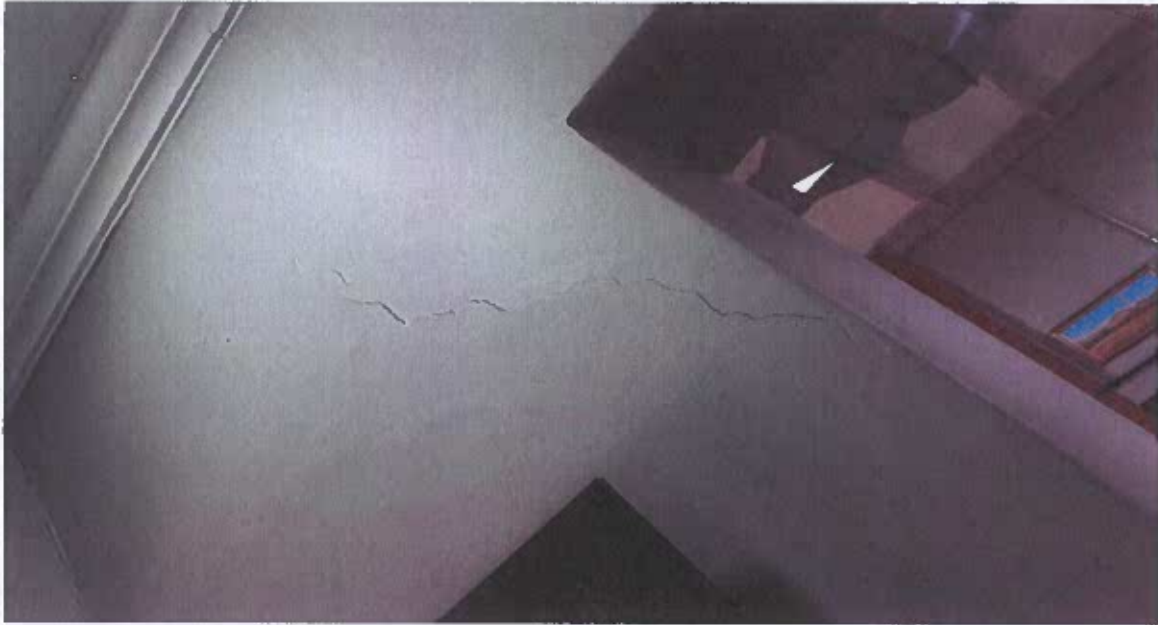
Plate 7 shows the recurrence of the repaired crack on the wall of the corrido.
