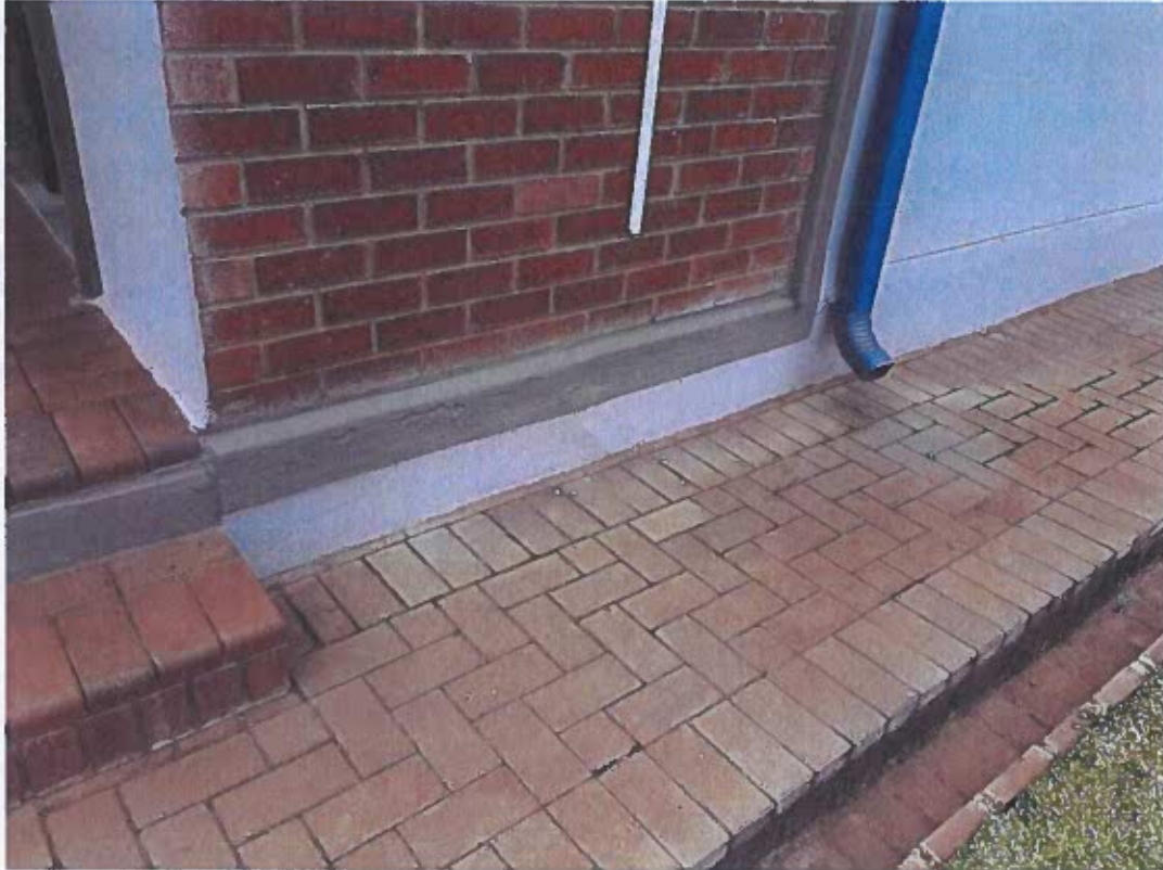
Plate 1 shows the signs of structural defects on the repaired western foundation wall.
