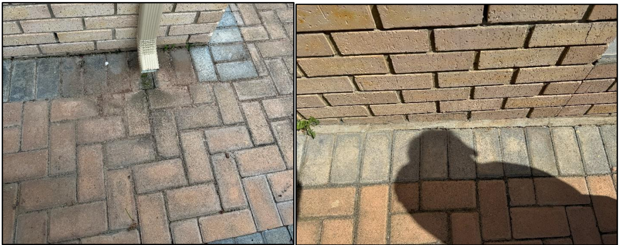
Figure 8: Showing the inadequate brick pavement with spaces between bricks around the house.
