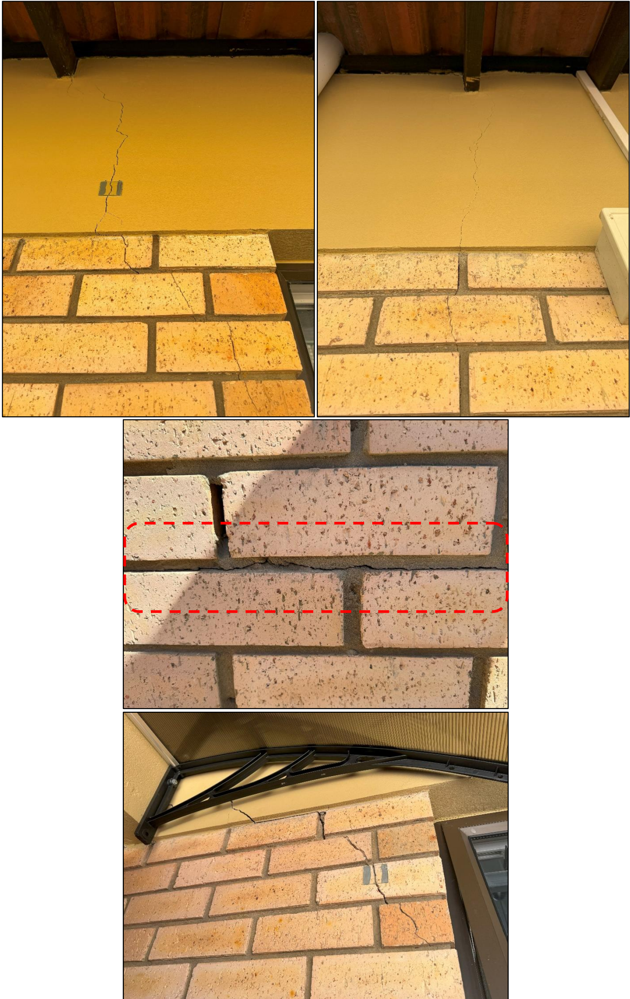
Figure 10: Showing the cracks on the exterior walls around the investigated house.
