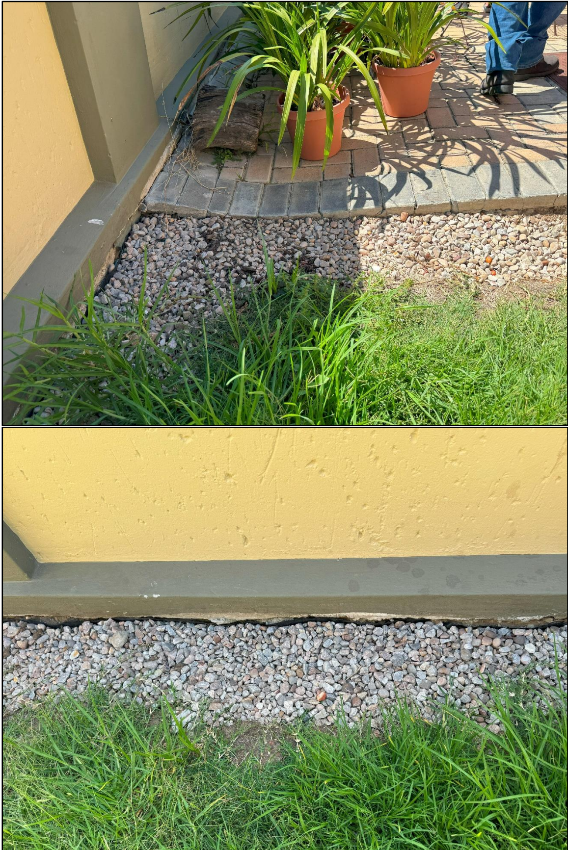
Figure 11: Showing the settlement in pavement and garden area.
