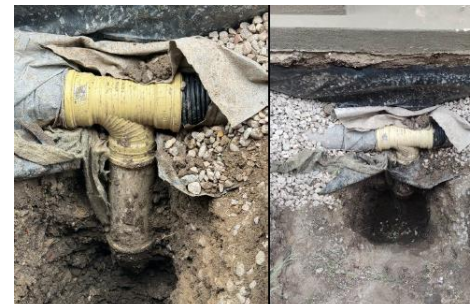
Sub-soil drain on eastern boundary
