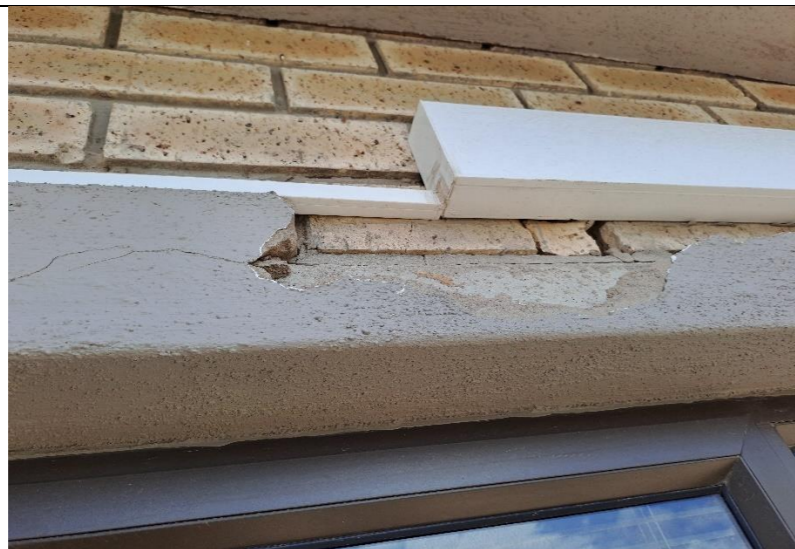
Photo 7: Cracks on external brick wall above window.
