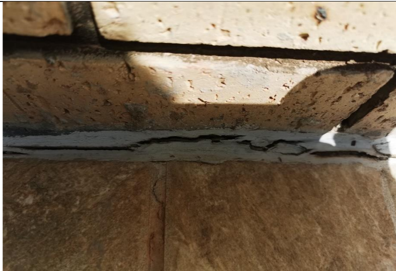
Photo 5: Delamination of joint sealant.
