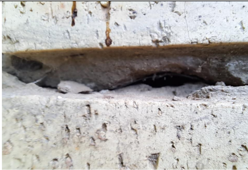
Photo 2: Bond mortar separation in-between the DPC and mortar course bed .
