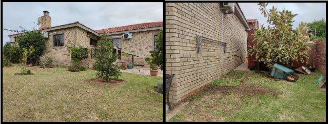
Figure 5: Showing the absence of a concrete apron on the north and the portion on the west side of the investigated house.
