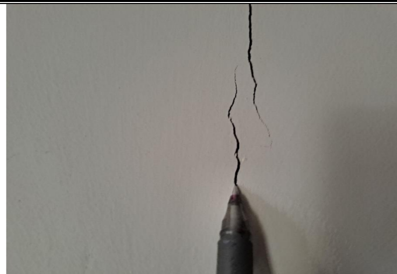
Photo 11: Vertical crack on internal wall.
