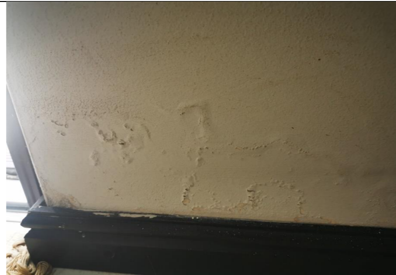
Photo 17: Dampness on internal brick wall.
