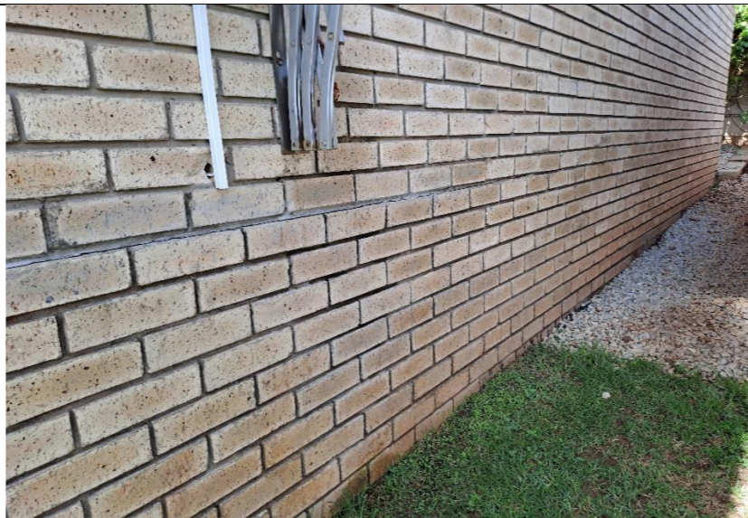
Photo 8: No aprons or stormwater around the building.
