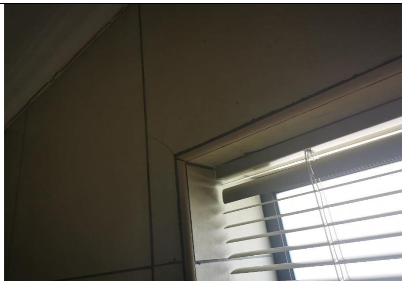
Photo 4: Diagonal crack on the internal bedroom wall above window.
