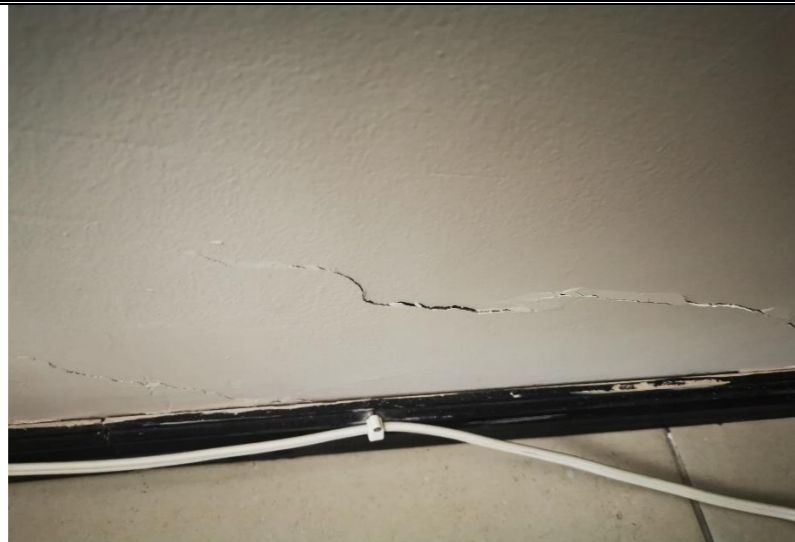
Photo 1: Vertical crack on internal wall.
