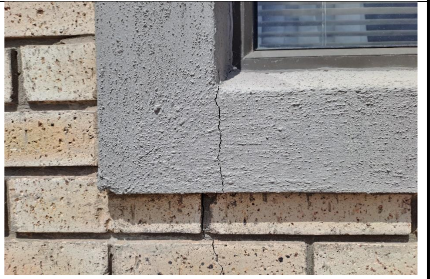
Photo 6: Crack on window seal
