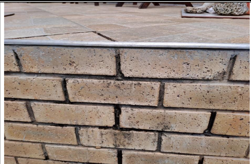
Photo 3: Algae and moulds has developed on the surface of the brick walls.
