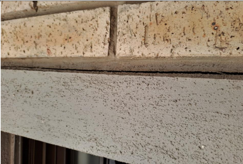
Photo 5: Horizontal crack above back entrance door.
