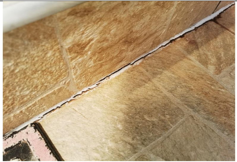
Photo 8: Delamination of joint sealant.
