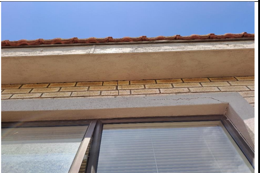
Photo 9: No roof gutters or rainwater downpipe.
