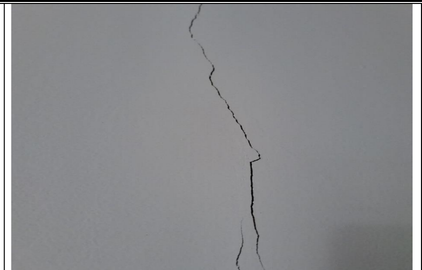
Photo 12: Vertical crack on internal wall.
