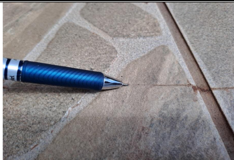
Photo 2: Cracks on floor tiles.
