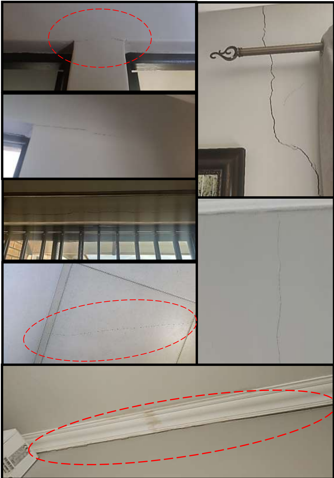
Figure 7: Showing the horizontal, vertical and diagonal cracks on the interior walls, floor and ceiling skirt around the investigated house.
