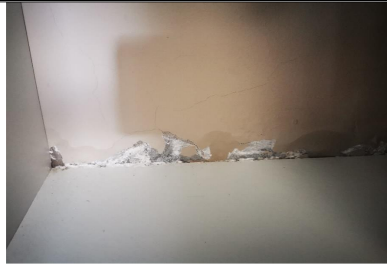
Photo 2: Dampness on internal brick wall.
