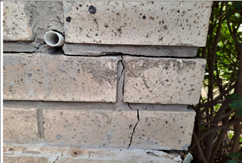
Photo 4: Horizontal crack at surface bed level .
