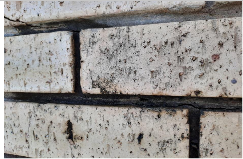
Photo 6: Algae and moulds has developed on the surface of the brick walls.
