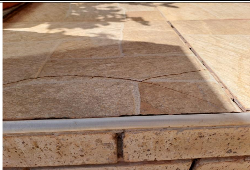
Photo 1: Cracks on floor tiles.
