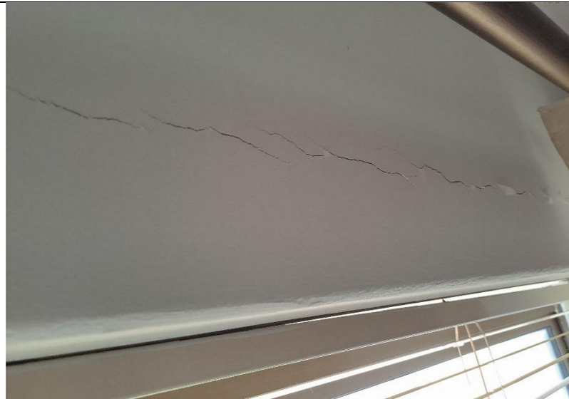
Photo 13: Horizontal crack above window.
