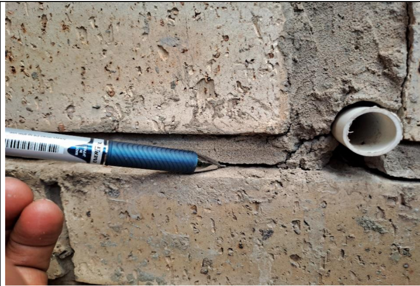
Photo 1: Horizontal crack at surface bed level
