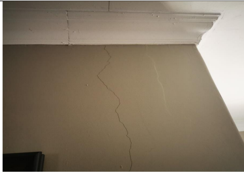
Photo 14: Vertical crack on internal wall.
