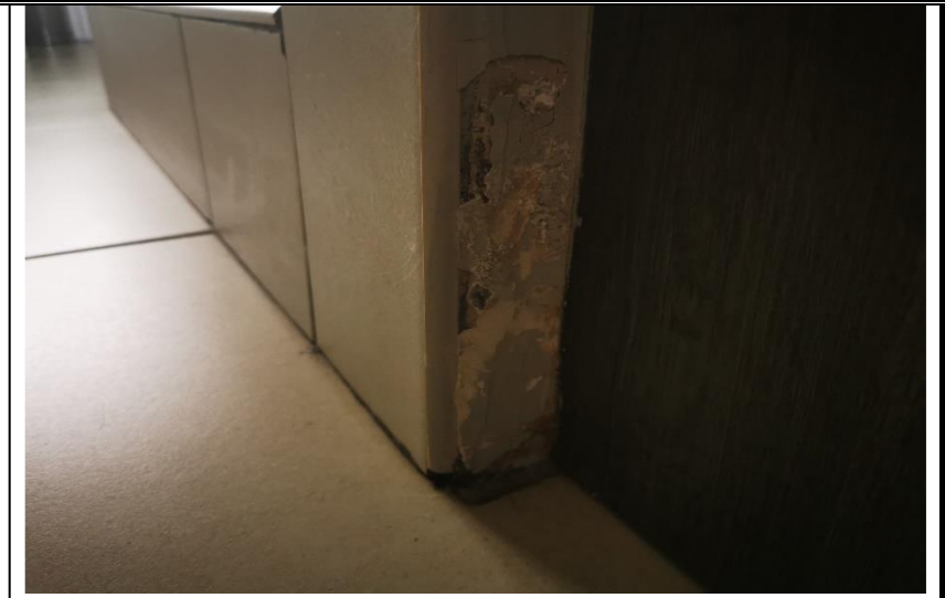
Photo 3: Dampness on internal brick wall.
