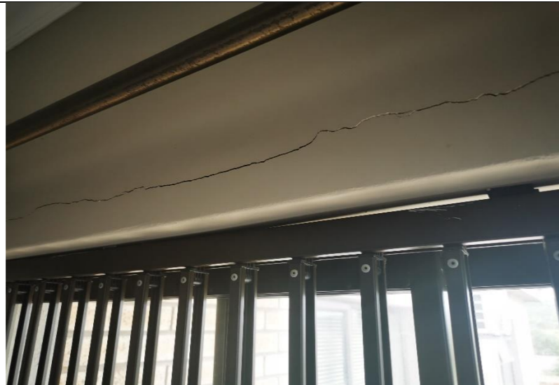
Photo 16: Horizontal crack above window.
