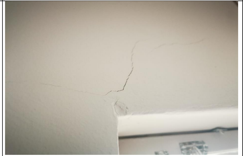
Photo 18: Diagonal crack on the internal bedroom wall above window.
