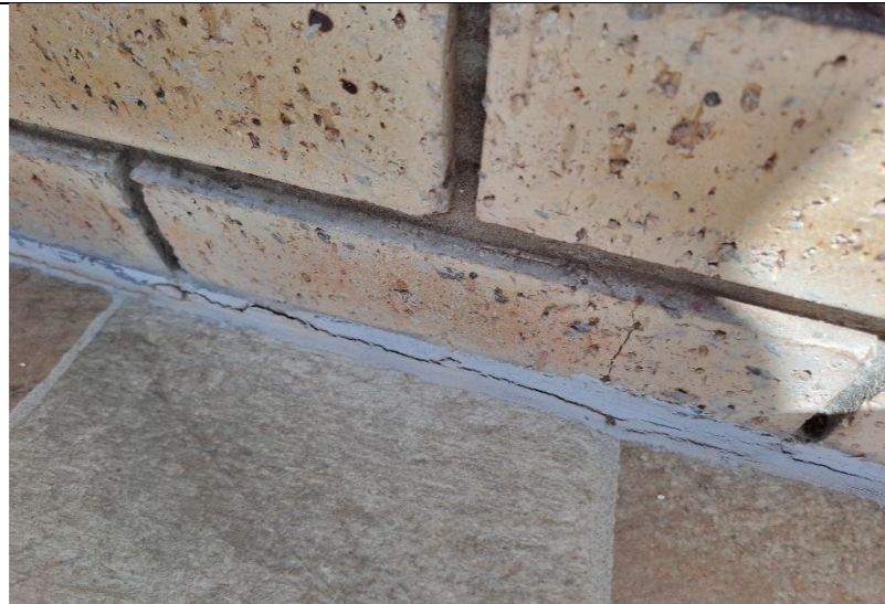
Photo 7: Delamination of joint sealant.
