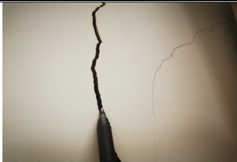
Photo 10: Major vertical-diagonal crack on the internal bedroom wall.
