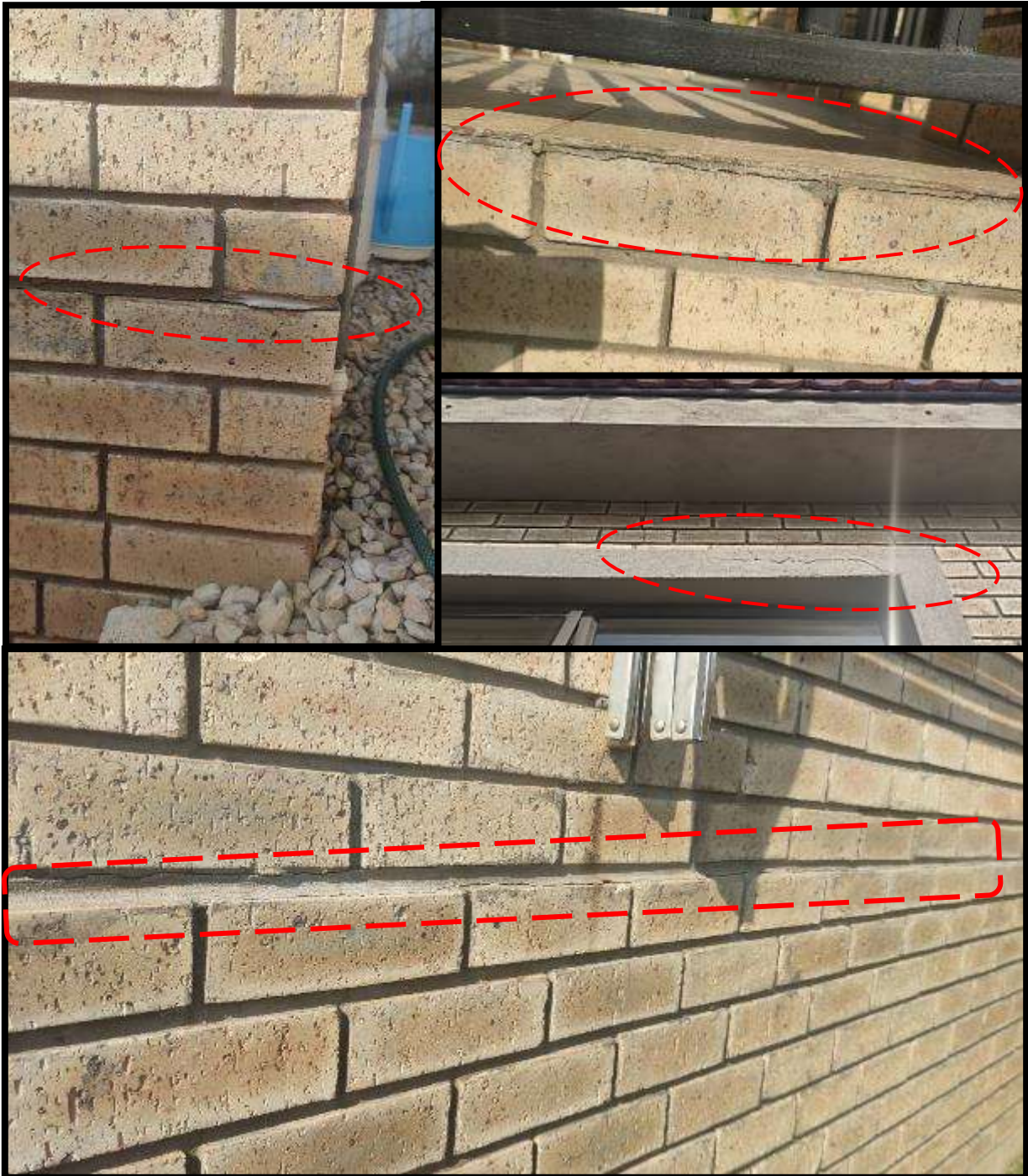
Figure 8: Showing the cracks on the exterior walls around the investigated house.
