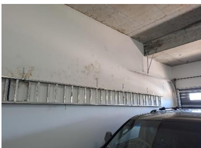
Pic 04: Water damp on the garage wall
