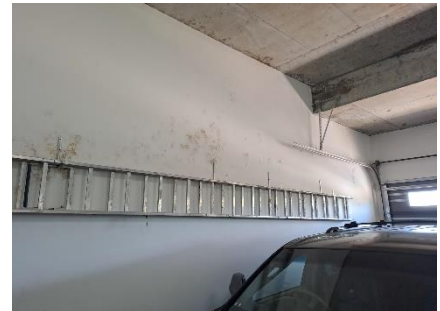
Pic 03: Water ingress on the garage walls
