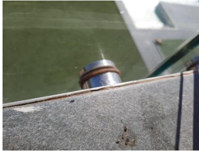
Pic 06: Tile edges not flush with tiles
