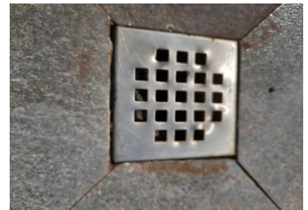
Pic 10: Poor waterproofing of the full-bore trap on the patio results in leaks to the living room
