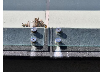
Pic 07: Water seepage - balustrade fixing bolts
