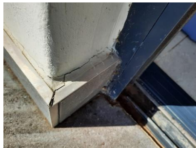
Pic 09: Blue coloured water seeping into cracks in walls and patio tiling
