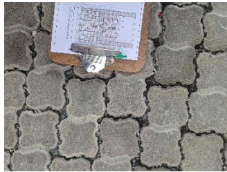
Pic 02: Large openings between segmented pavers.
