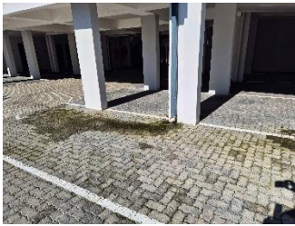
Pic 01: Rainwater ponding at down-pipe locations.
