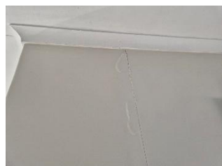
Pic 17: Crack at movement joint with plaster peeling off.
