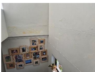
Pic 21: Water damp against wall and division of 4 th and 3 rd Floor.
