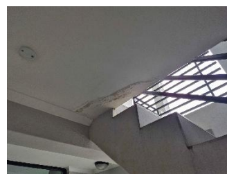
Pic 06: Water seepage and cracks in staircase slab.
