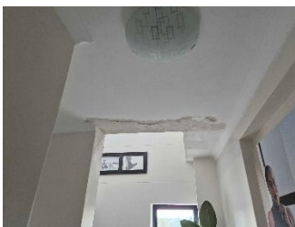
Pic 05: Water seepage and cracks – Unit 16
