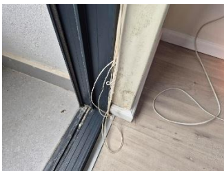
Pic 09: Unit 14 – Balcony level higher than inside FFL.
