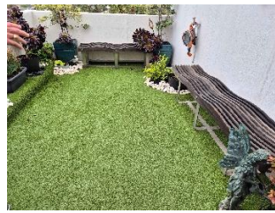
Pic 15: Soaked southern patio, no drainage with blocked outlet.
