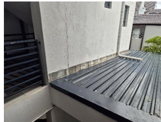
Pic 03: Weepholes blocked and roof cladding coming loose.
