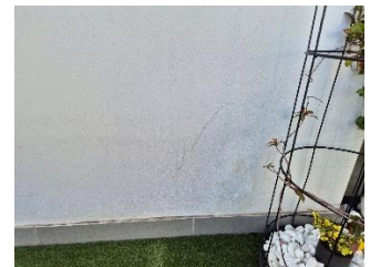
Pic 16: Water damp and crack against wall.
