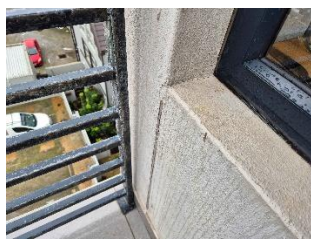
Pic 14: Cracks in wall at expansion joint, water ingress.
