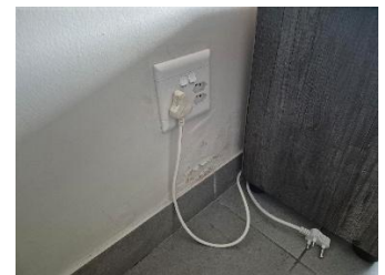
Pic 12: Water ingress dangerously near electric plug
