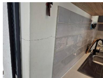
Pic 07: Structural crack in kitchen wall.
