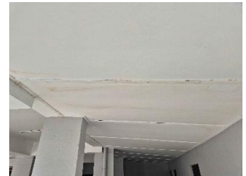
Pic 04: Water damp collecting on soffit of parking roof.
