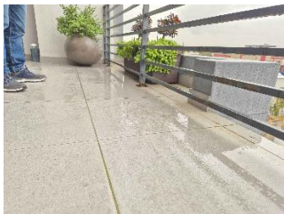
Pic 13: Standing water on southern patio, no drainage.
