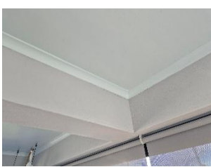
Pic 18: Water damp and crack against beams and ceiling.
