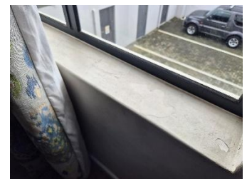
Pic 08: Water damp collecting on window sills.
