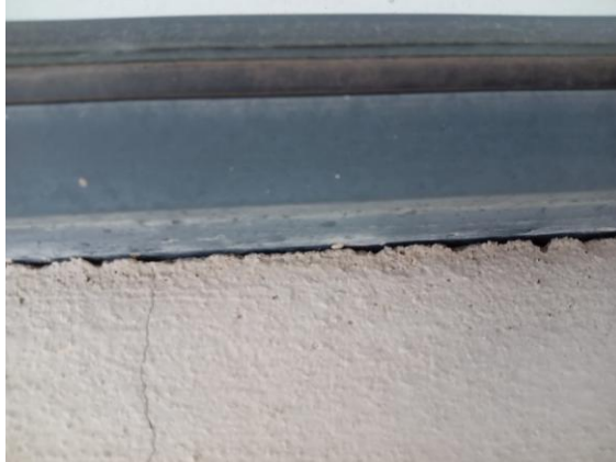
Figure 10: Aluminium Window and Plaster Separation
