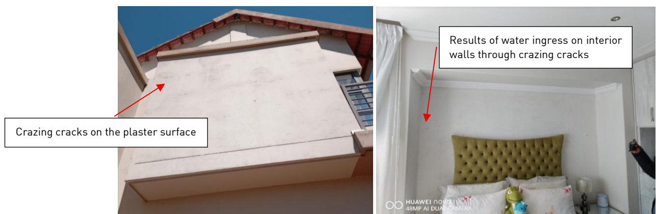
FIGURE 5: PLASTER CRACKS ON BEDROOM WALL
