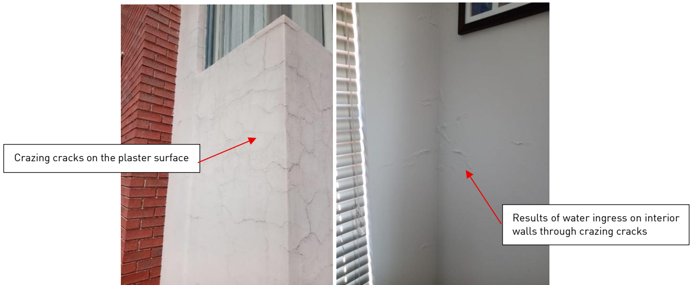
Figure 4: Exterior Plaster Cracks
