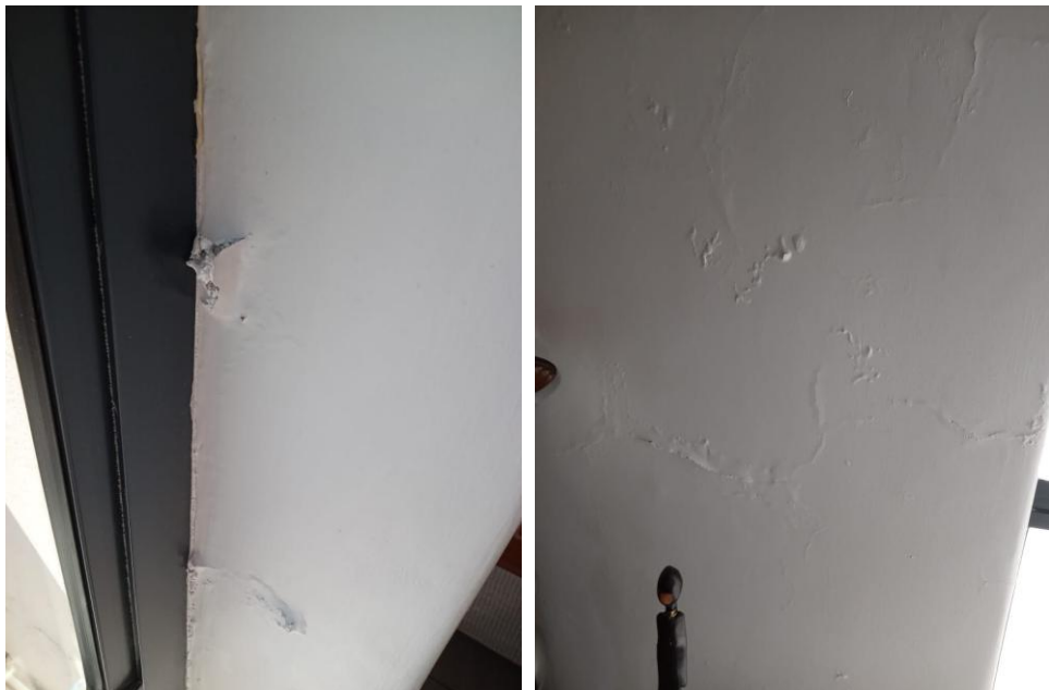
Figure 11: Interior Plaster Damp and Calcium Build Up Due to Water Ingress
