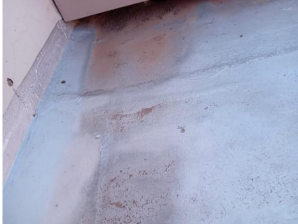
Figure 15: Incorrectly Sloped Screed at DP 2
