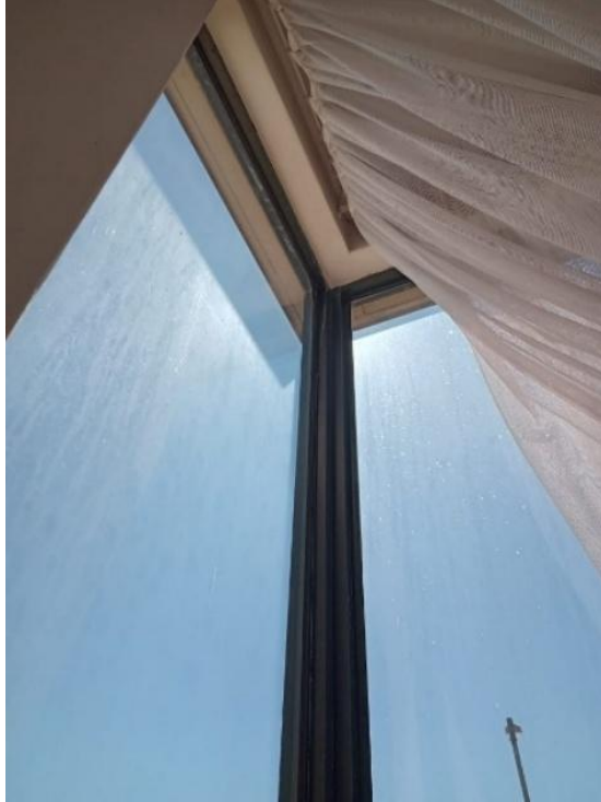
Figure 12: Leaking Aluminium Windows
