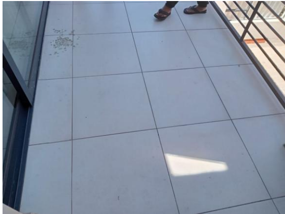
Figure 8: Balcony 1 with Insufficient Slope
