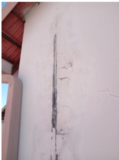
Figure 7: Water Pipes Inadequately Installed
